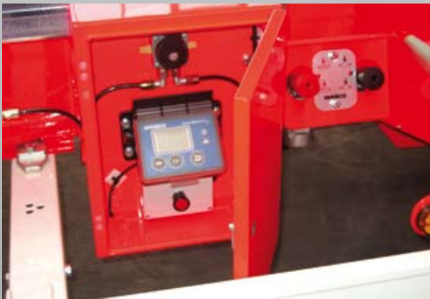
Function switch in protective box
